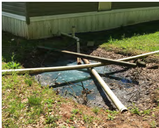
Straight piping sewage to ditch behind home in Lowndes County, Alabama. Photo Credit: DOJ/Civil Rights Division
