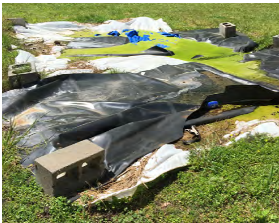
Covered sewage ditch in Lowndes County, Alabama. Photo Credit: DOJ/Civil Rights Division
